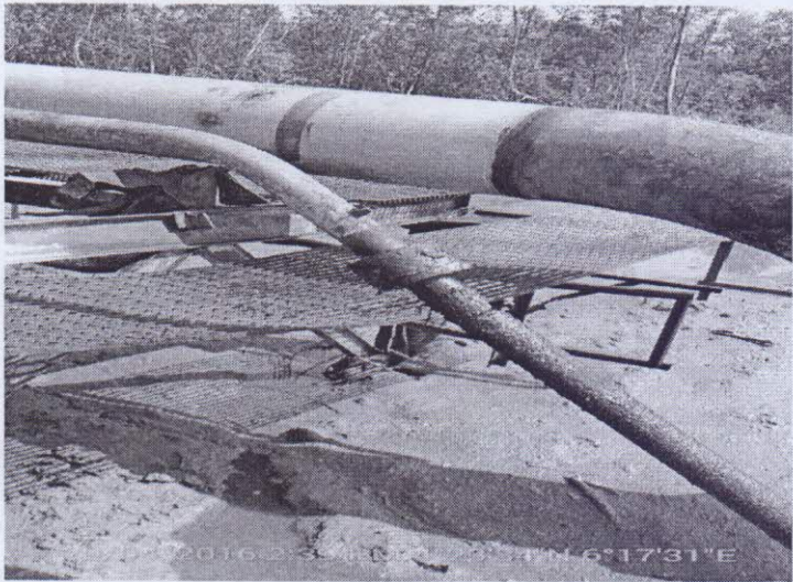
POINT BEFORE REPAIR: fig1
